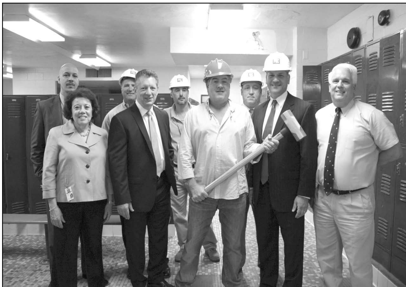
School and construction officials break ground for the new locker rooms at Glen Cove High School on June 3. The renovations will include new floors, ceilings, lockers and showers, all in school colors to give students a strong sense of school pride.
