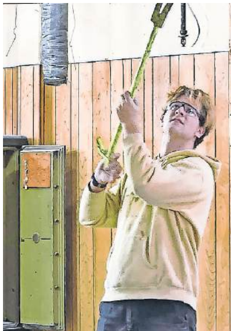
Oliver Schweiger spent most of the day taking measurements and tearing down walls during last December's demolition.
