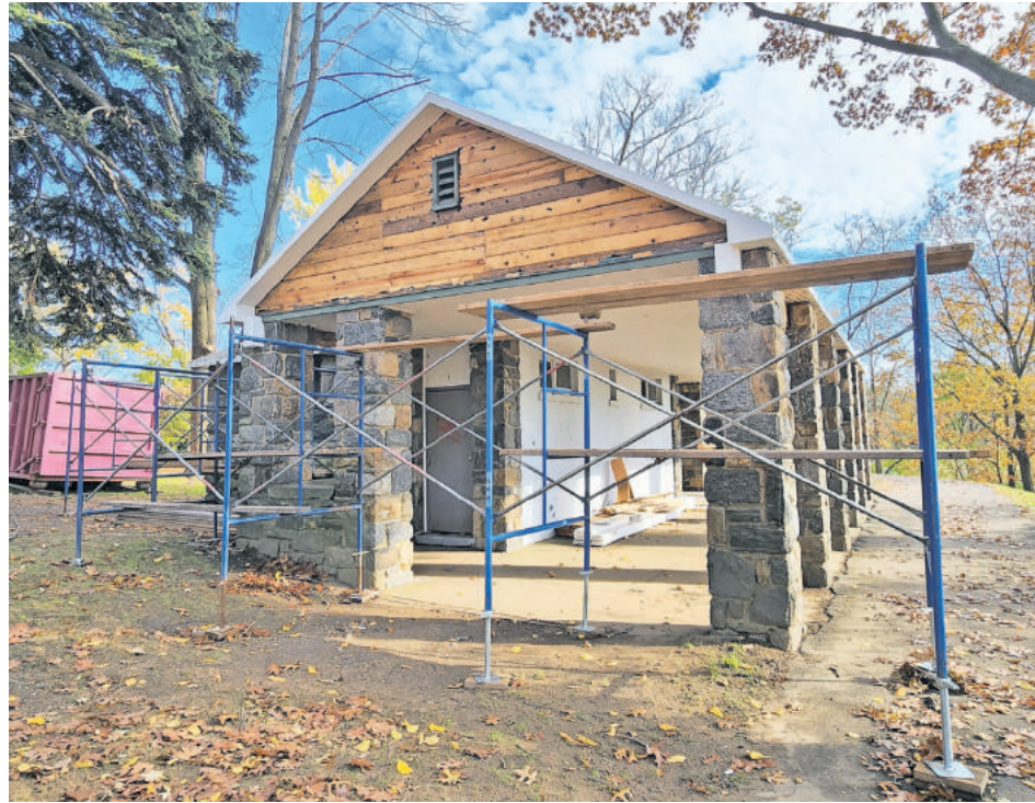
MORGAN PARK'S UPPER bathhouse is currently under renovations. The building needs extensive repair to its roof and plumbing.
