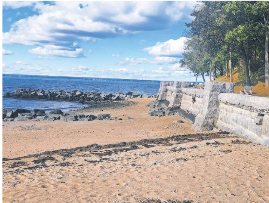
The seawall is deteriorating, and the project will reinforce it with rapid-setting concrete, and replace the failing brick in the pavilions with new masonry.
